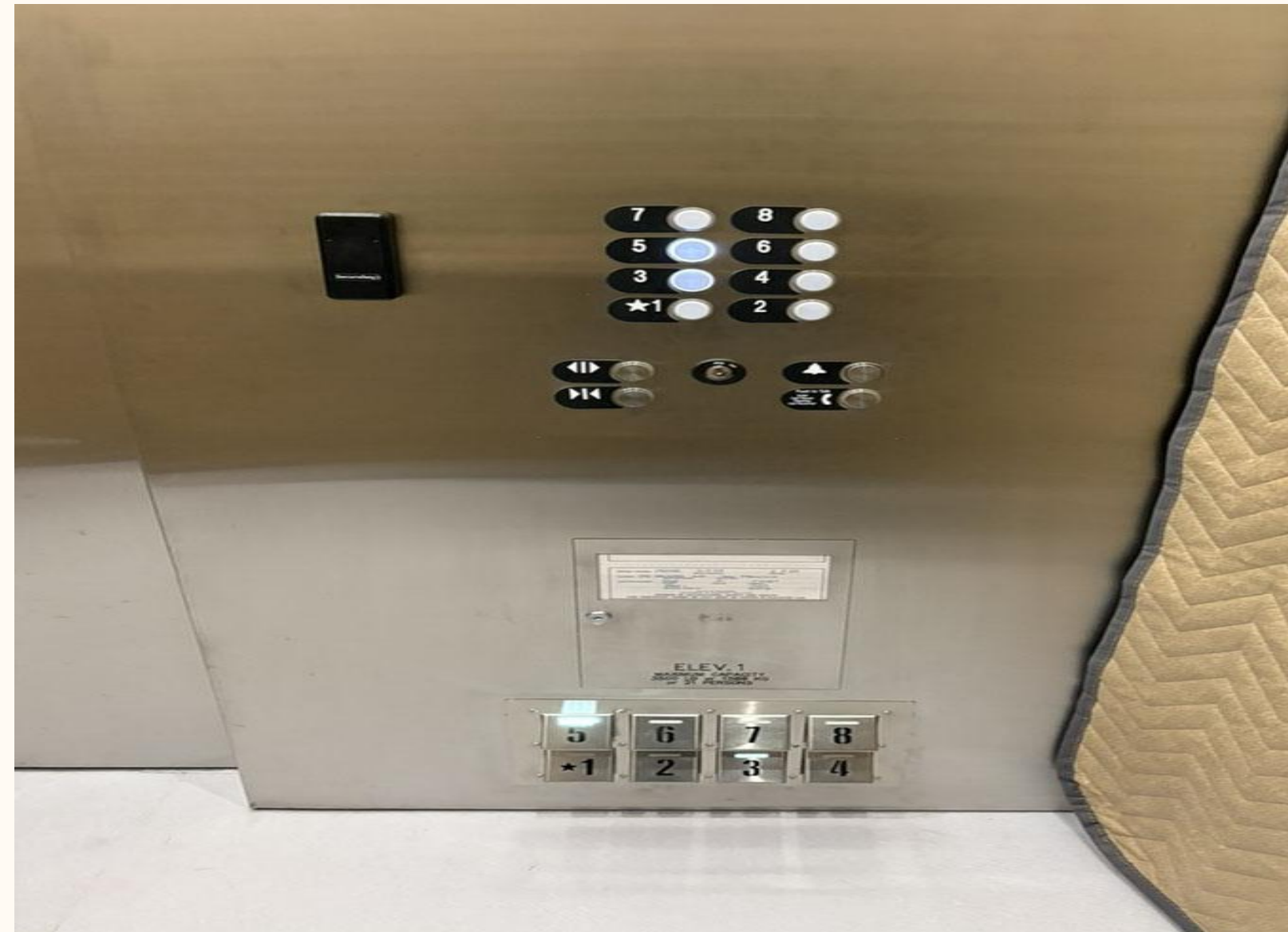
Elevator Foot Controls
